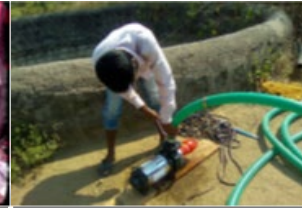
Water Pump Installation
