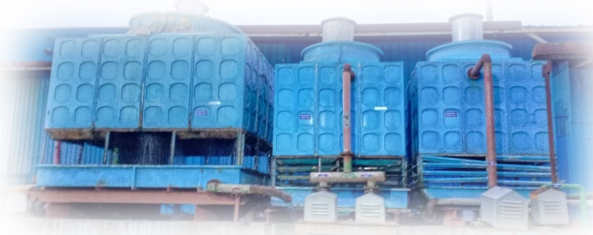
Cooling Tower @ our Conductor Plant
