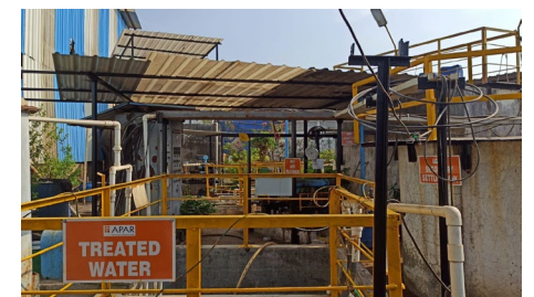
STP facility @ our Cable Plant
