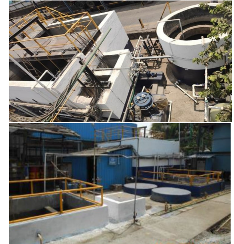
ETP facility @ our Oil Plant
