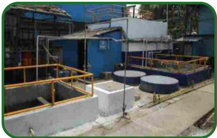
ETP plant at Rabale, Navi Mumbai
