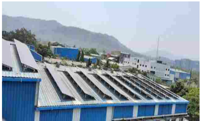
Solar Panels on White Oil Plant @ Rabale (Navi Mumbai)
