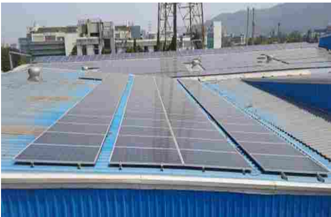
Solar Panels on A&I Plant @ Rabale (Navi Mumbai)
