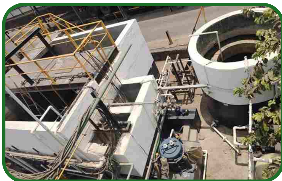
ETP plant at Rabale, Navi Mumbai
